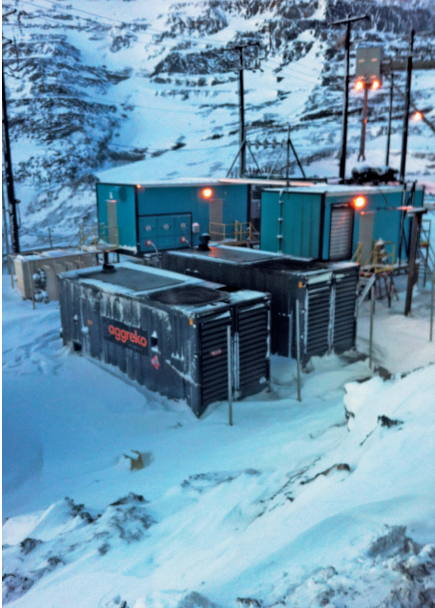
Aggreko Canada has been seeing increased demand for temporary power solutions, such as this 5 MW solution for Grand Cache Coal
