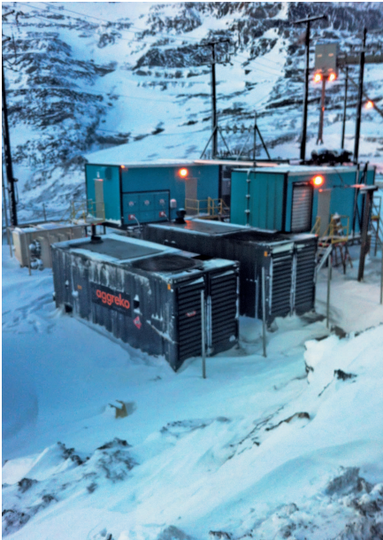
Aggreko Canada has been seeing increased demand for temporary power solutions, such as this 5 MW solution for Grand Cache Coal
